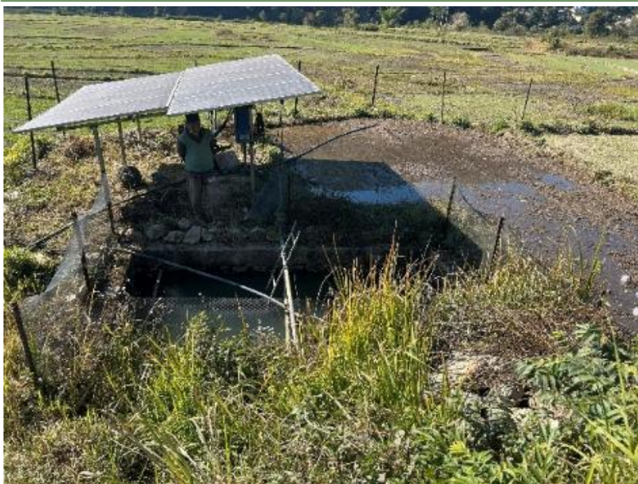
The solar-powered submersible pump installation at Rampur's water source.
