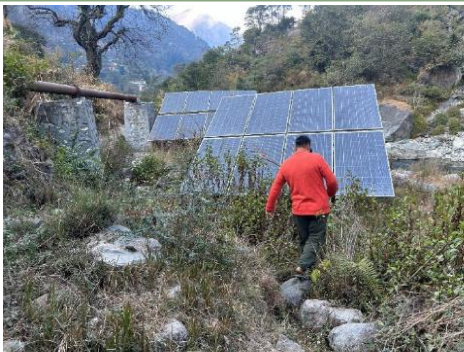
Solar panels installed above the Asiganga river at Simoldi.
