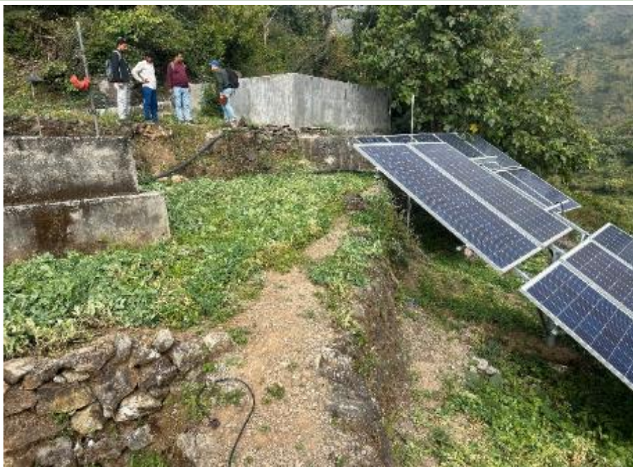
RCC storage tanks and solar panels installed above Kyara-Badait village.
